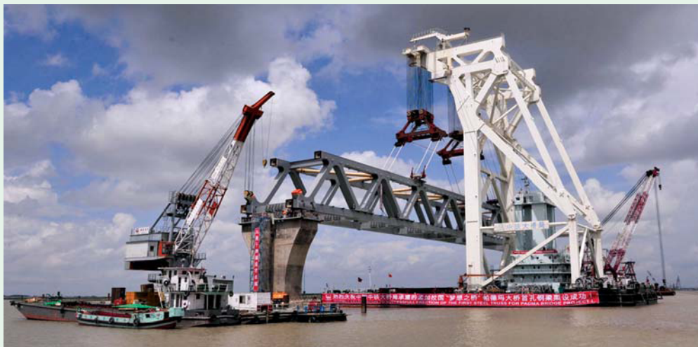
Installation of the first span of the Padma Bridge at the Zanjira point in Shariatpur, September 30
